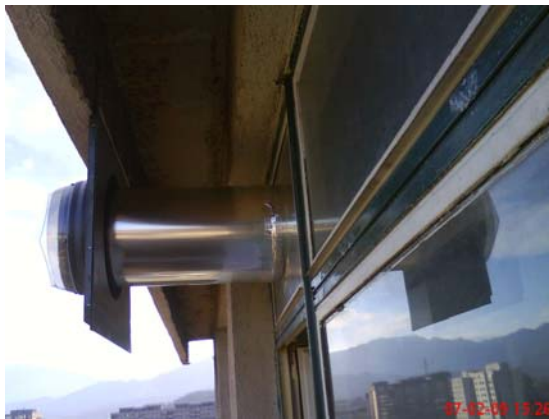
Figure 3 Daylight dome collector of the horizontal SunPipe installed on the façade.
