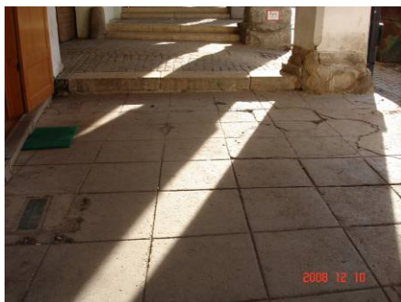
EXISTING SITUATION - ACCESS, Asymmetric and chaotic lighting, with LED reflectors
