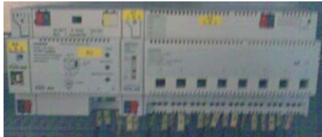
Figure 8 KNX simple ensemble (Source+line coupler+load switch)
