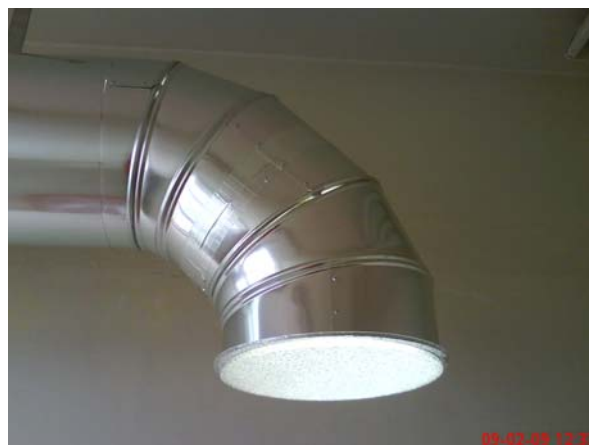
Figure 15 Internal end of the horizontal SunPipe.
